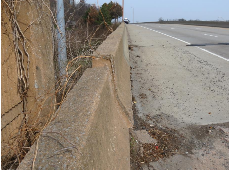
BRIDGE PARAPET "B" END RT. MISALIGNED
