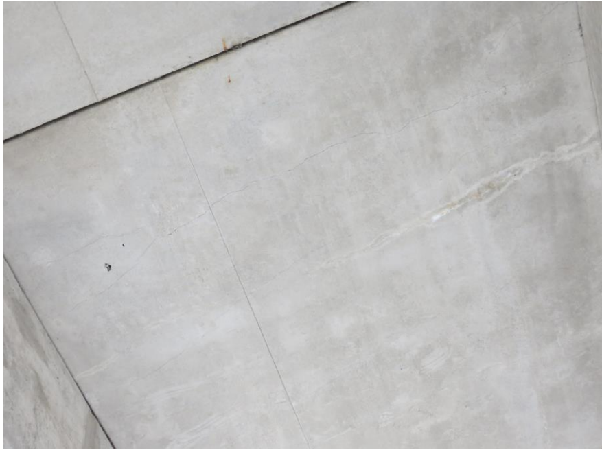
DECK PANEL BAY "C" SP. #3 W/ TRANSV. CRACK
