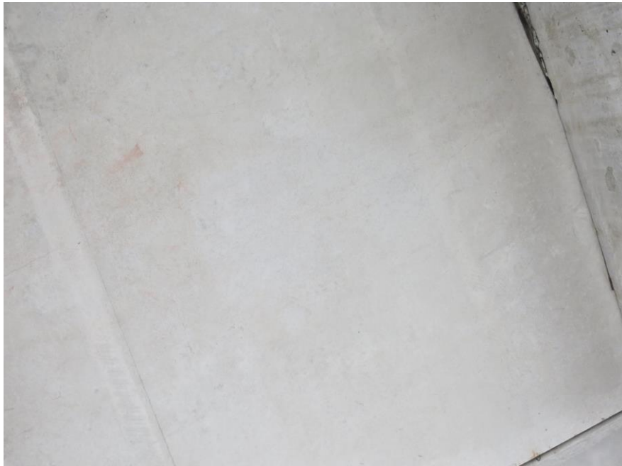
DECK PANEL BAY "B" SP. #3 W/ TRANSV. CRACK
