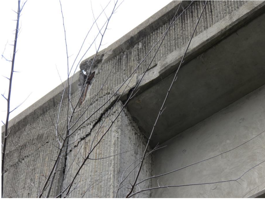
BRIDGE RAIL "B" END LT. W/ IMPACT DAMAGE
