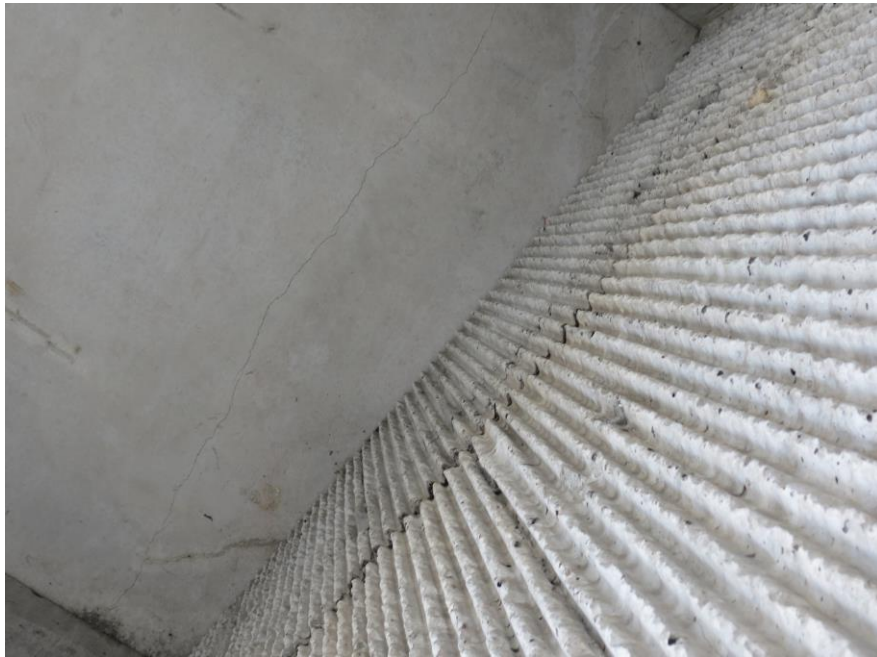
DECK PANEL BAY "A" SP. #3 W/ TRANSV. CRACK
